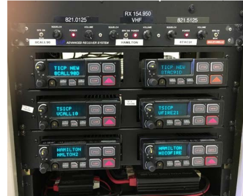
Figure 4-4: Hamilton County Sheriff's Office Control Stations
